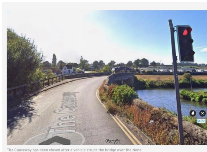
The Causeway has been closed after a vehicle struck the bridge over the Nene
